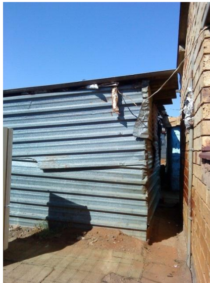
Figure 4: The Ndala house has expanded, with outside corrugated iron extensions that house tenants Photo: Lindiwe Mbongwe, 2012
